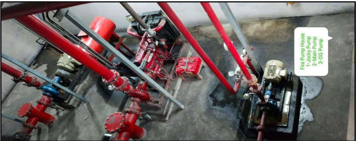
Fire D.V System
